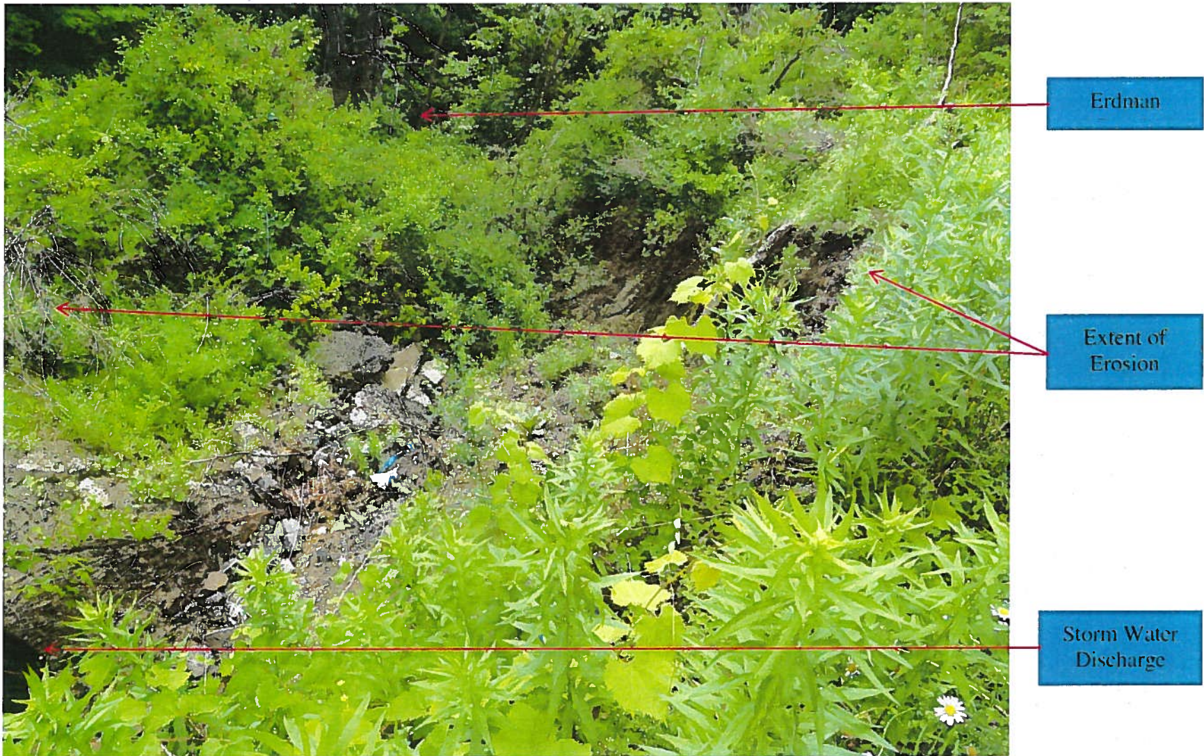
Figure 4. Erosion at storm water outfall S-09, looking down slope from the top of the Lagoon 3 embankment.
