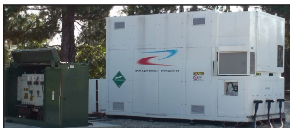
Zenergy fault current limiter operating in Southern California Edison's Avanti Circuit
