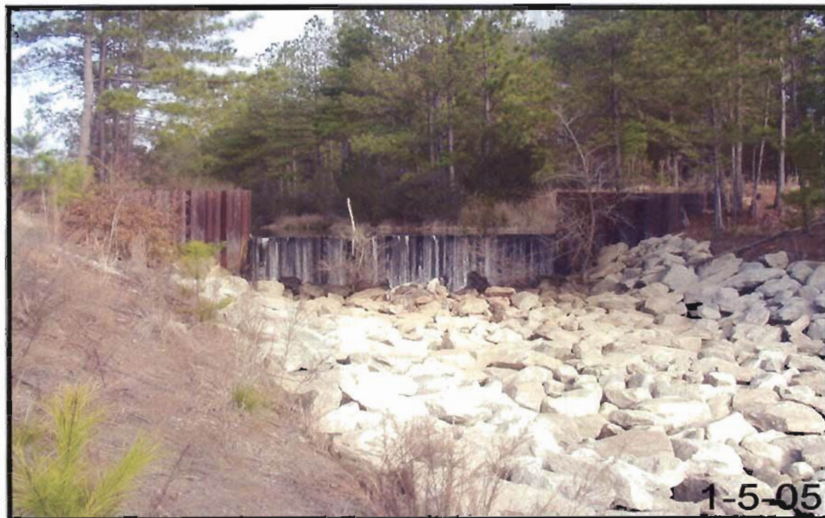
Figure 2-13. View of Proposed New Location for Outfall F-08 at Downstream Sheet Pile Dam.
