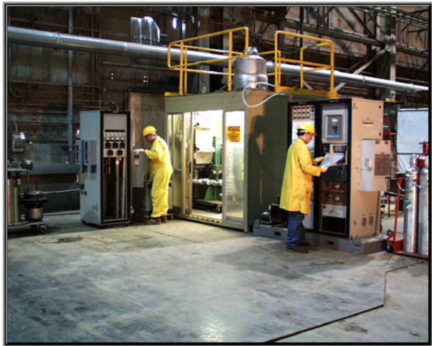
MOLTEN SALT OXIDATION UNIT
