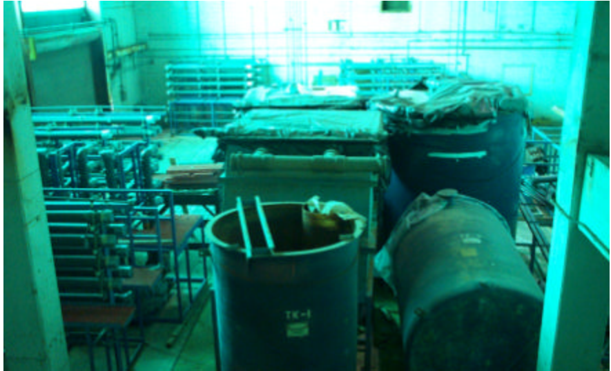
CONTAMINATED WASTE WATER TREATMENT PLANT AT RMI METALS FACILITY
