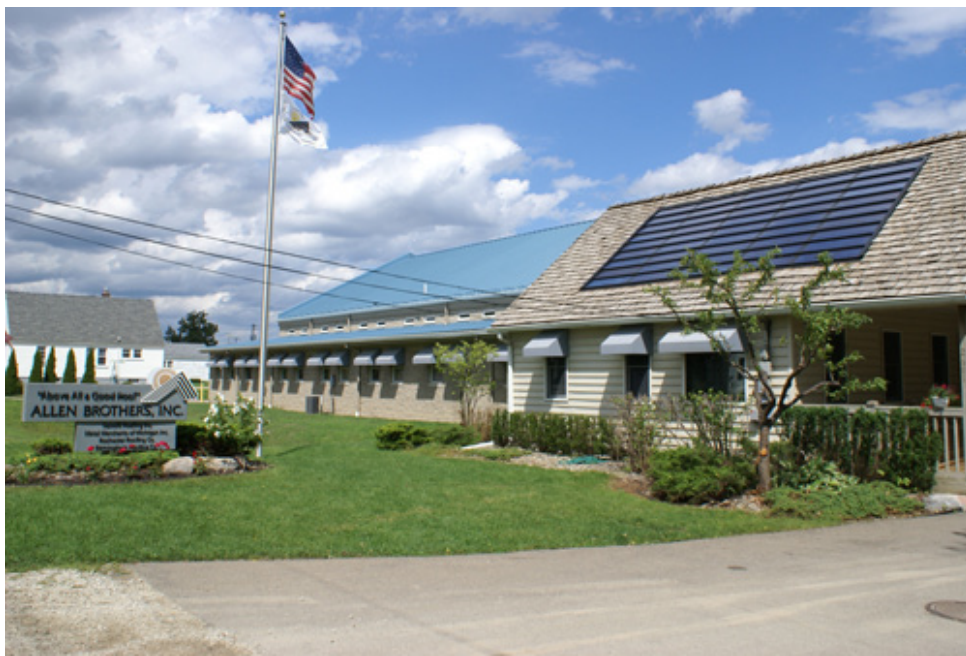
The Allen brothers have installed their BIPV product on the roof of their Rochester Hills headquarters. | Photo courtesy LUMA Resources
