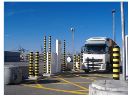
NNSA's Second Line of Defense Megaports Initiative installation of portal monitors at Antwerp in Belgium to detect illicit trafficking of nuclear and radiological material.
