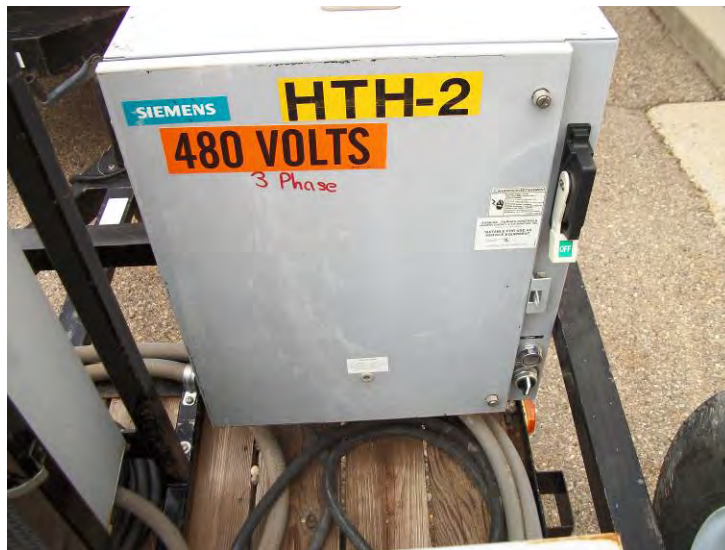
Figure 4. Typical Disconnect Switch
