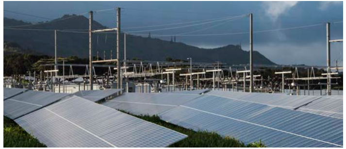
AES Lawai Solar Project- Kauai Photo by Dennis Schroeder / NREL 58020
