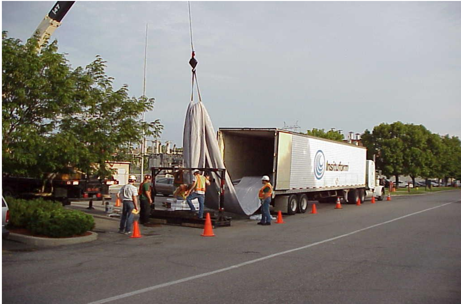
INSTALLATION OF NEW LINING FOR A SUBSURFACE SITE DRAIN AT KANSAS CITY PLANT
