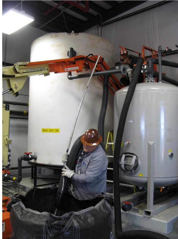
GRANULAR ACTIVATED CARBON FILTER MEDIA CHANGE-OUT AT PANTEX PLANT
