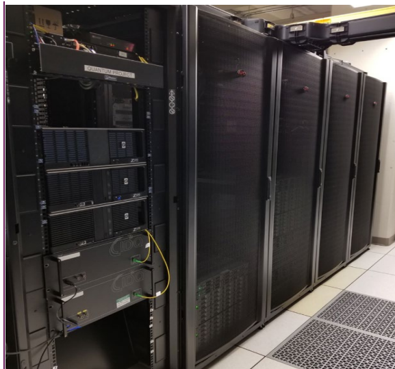
Quantum communication terminals installed in EPB’s Chattanooga substation.
