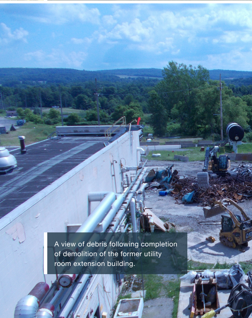
Workers begin demolishing a former utility room extension building at EM's West Valley Demonstration Project. It was one of seven support buildings of the Main Plant Process Building. Three of those structures remain and are scheduled for demolition.
