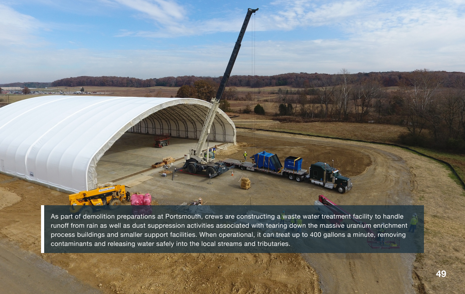
The On Site Waste Disposal Facility (OSWDF) is currently under construction. The OSWDF is specifically engineered and built to safely accept contaminated debris from the gaseous diffusion buildings at Portsmouth.
