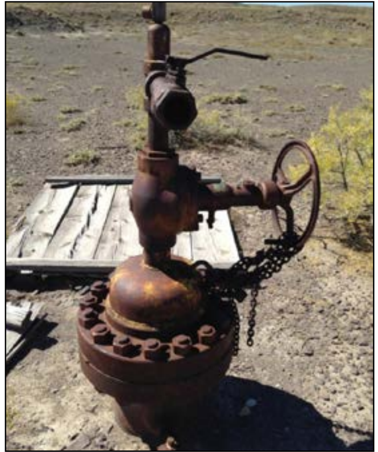
Utah, Utah, Site Wellhead, Looking South, September 27, 2016
