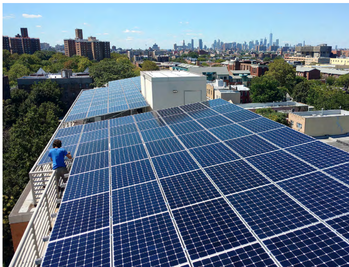
A rooftop solar PV array on a multifamily apartment building in Brooklyn, New York. Photo credit Bright Power, Inc.
