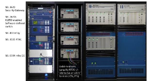
Real-Time Distributed Control system used for initial controller demonstration
