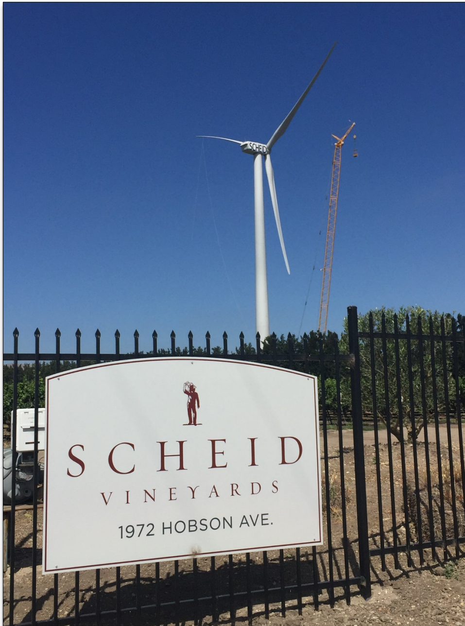
The Scheid distributed wind installation is Foundation Windpower's third Salinas Valley project. Photo by Foundation Windpower, LLC
