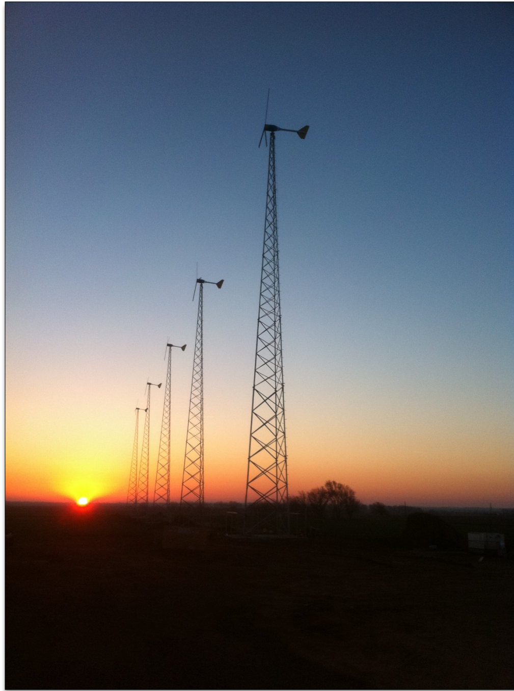
The Drummond turbines are installed on 120-foot self-supporting towers. Photo by Pieter Huebner
