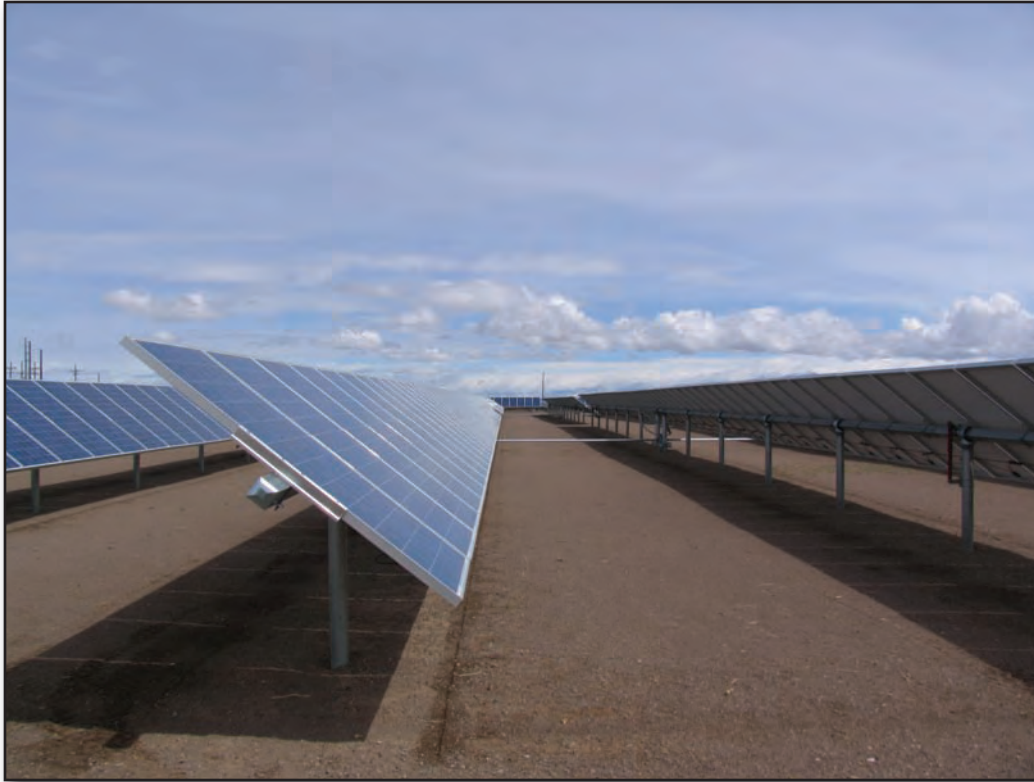
Fixed-axis photovoltaic panels at the Alamosa photovoltaic power plant near the New Mexico border (NREL).
