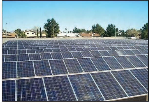
Figure B-6. Ground mounted PV system, Ronzone Reservoir, Nevada (Sunpower Corporation).
