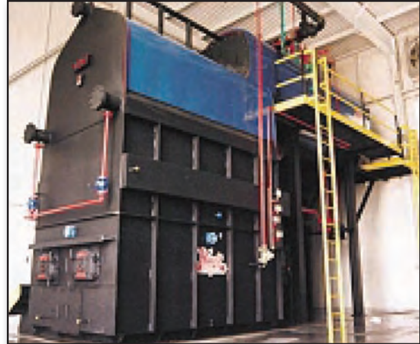
Figure 5.4-3. Typical 38 MMBtu biomass boiler.
