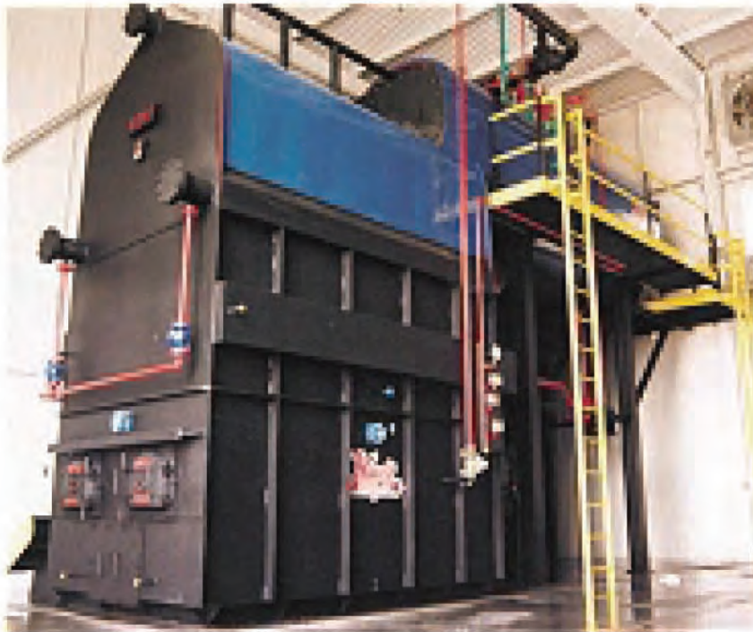
Picture 1: Typical 38 mmBtu boiler
