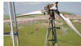
Photo by Shawn Smallwood, NREL 17329
