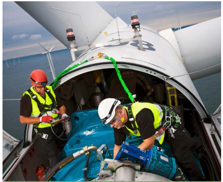
Photo from Siemens AG, NREL 19687
