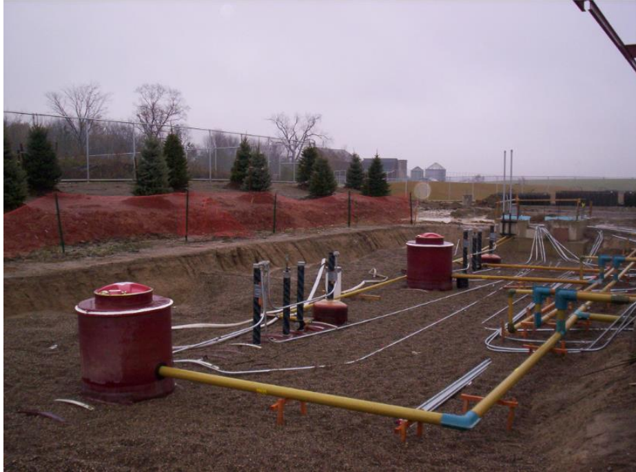
Figure 2-4. The Underground Storage Tank System After Gravel Cover and Prior To Driveway Installation. Photo Source: Oscar W. Larson Co., Clarkston, MI.
