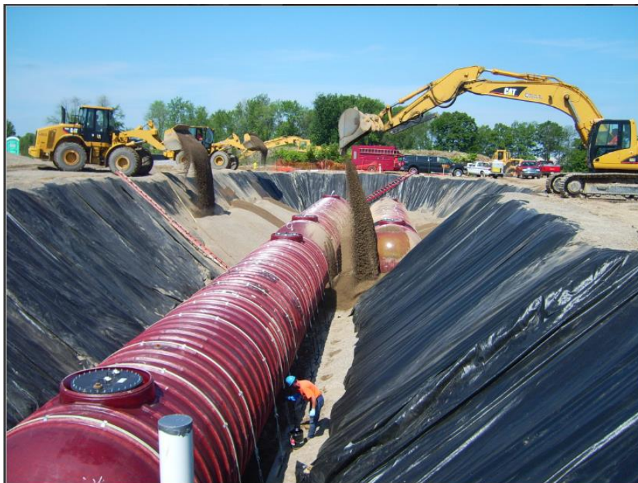
Figure 2-3. The Underground Storage Tank System Being Covered Prior To Driveway and Line Installation. Photo Source: Oscar W. Larson Co., Clarkston, MI
