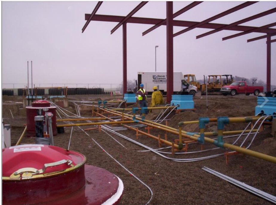
Figure 2-5. The Underground Storage Tank System After Line Installation Prior To Driveway Installation. Photo Source: Oscar W. Larson Co.
