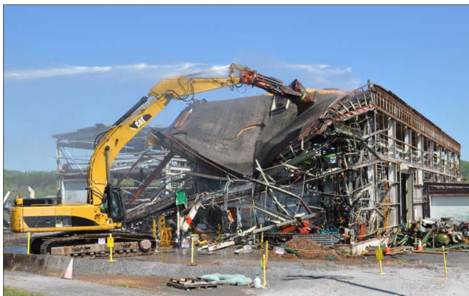
Crews began tearing down Building K-633 in May and completed the project in June.
