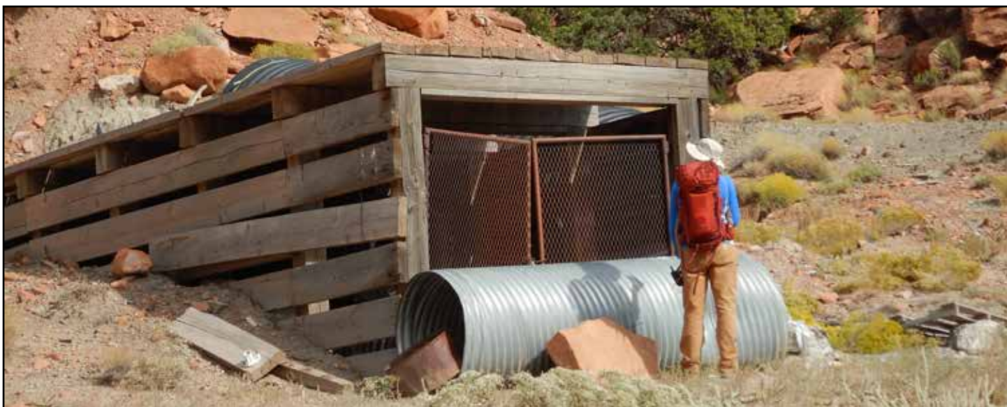
Bulls Eye Mine gated adit with snow shed and vent pipe, Red, White, and Fry Canyons and Deer Flat Districts, Utah, BLM-administered public land.
