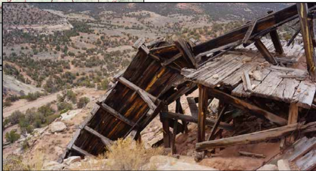
Tramp Mine unstable ore chute, Uravan District, Colorado, BLM-administered land.
