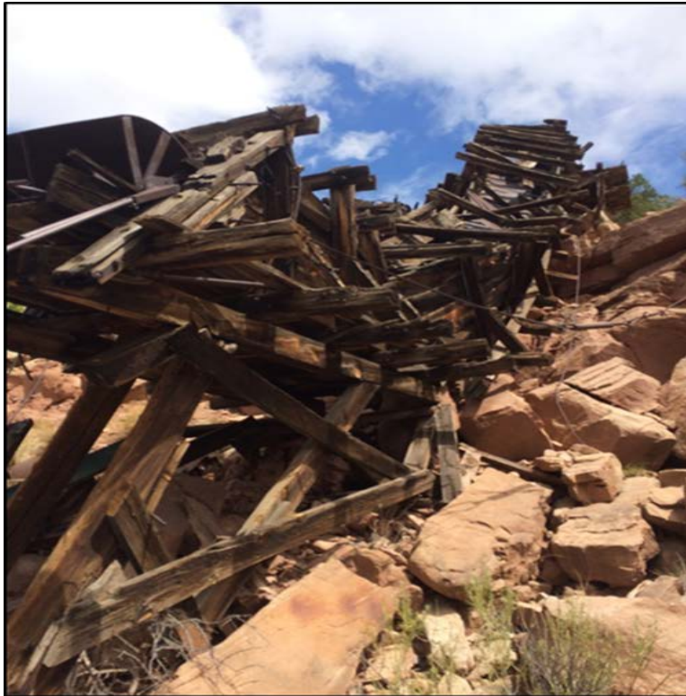
Figure 7. Collapsed Wooden Ore Chute at the Tramp 2 Mine, Club Mesa, Colorado
