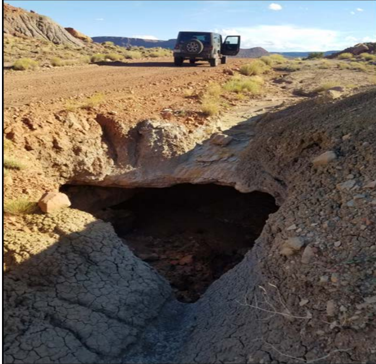
Figure 9. Daisy 2 Mine, Large Subsidence Feature next to the Road, Red Canyon, Utah
