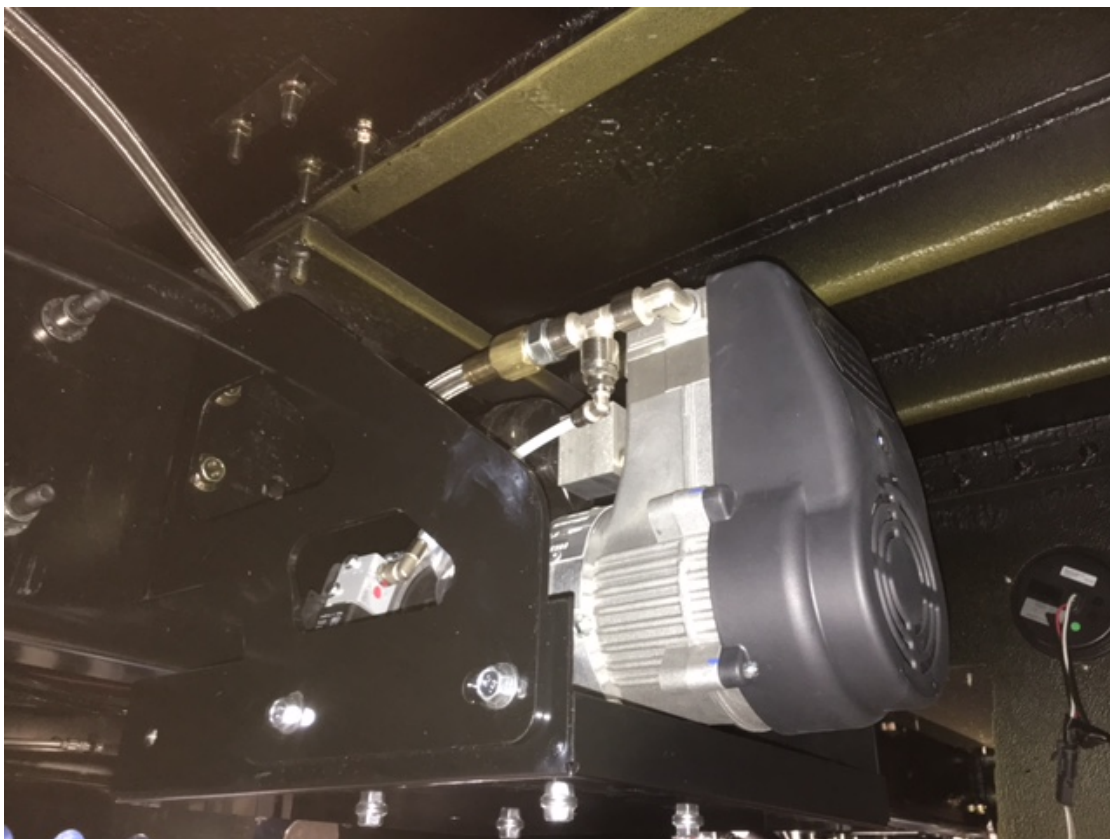
Figure II.5.2 - Air Compressor Installation in Bus P1
