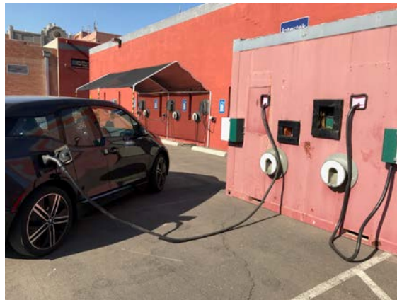
Figure III.6.3 - A 2014 BMW i3 BEV DC fast charging using the StAR unit (enclosed in red chamber) at Intertek in Phoenix, Arizona/Intertek
