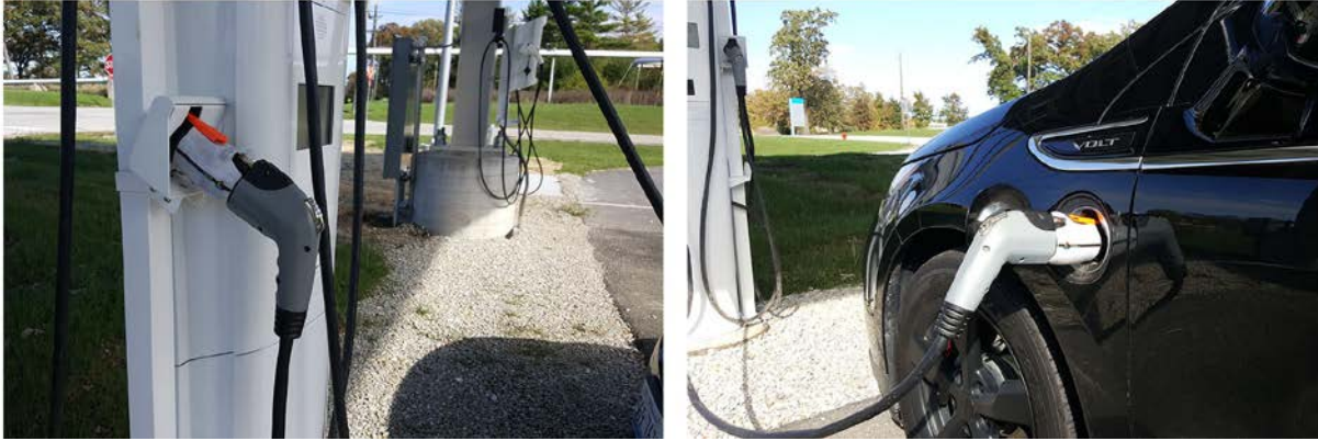
Figure V.1.2 - ANL SCA locked to a public EVSE and connected to a GM Volt while charging (Source: ANL)
