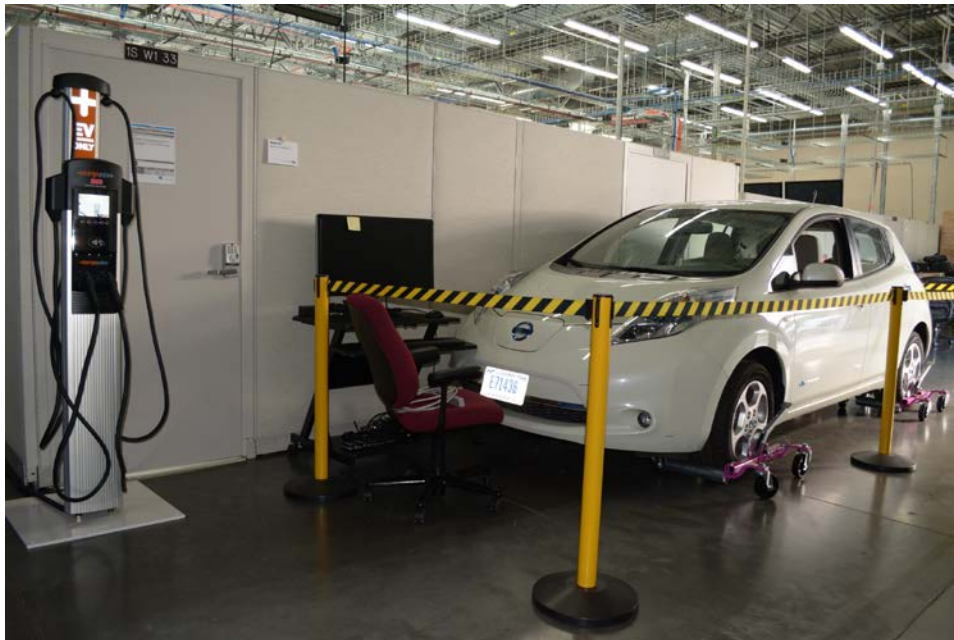
Figure IV.4.2 - Vehicle Development Lab - PEV, EVSE, and BEMS Station
