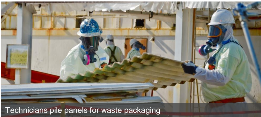
Transite panels are removed from the east face of the C-410 Feed Plant
