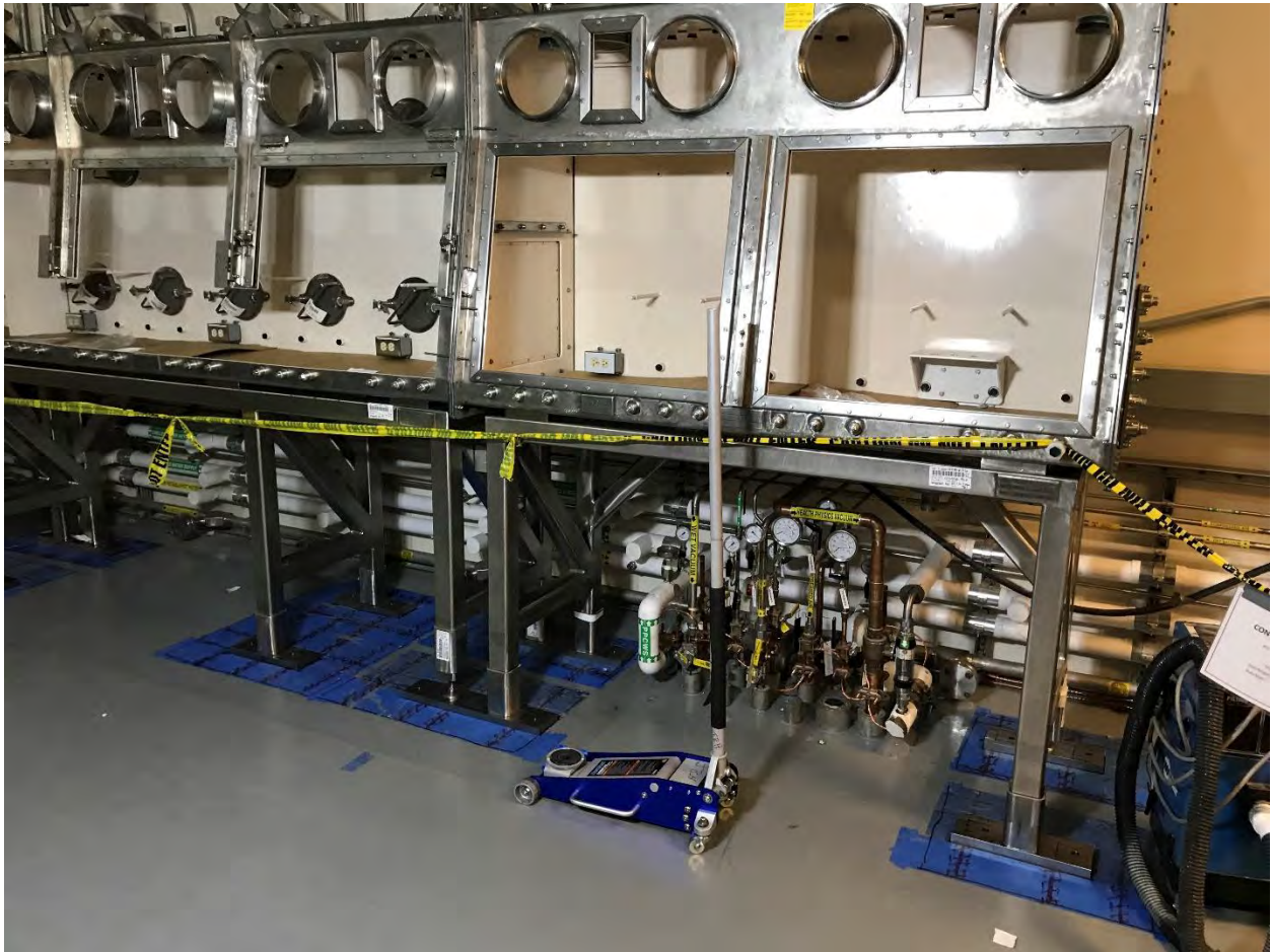
Installation of Ventilated Enclosure and Utilities for Analytical Chemistry Analysis in RLUOB (2017)
