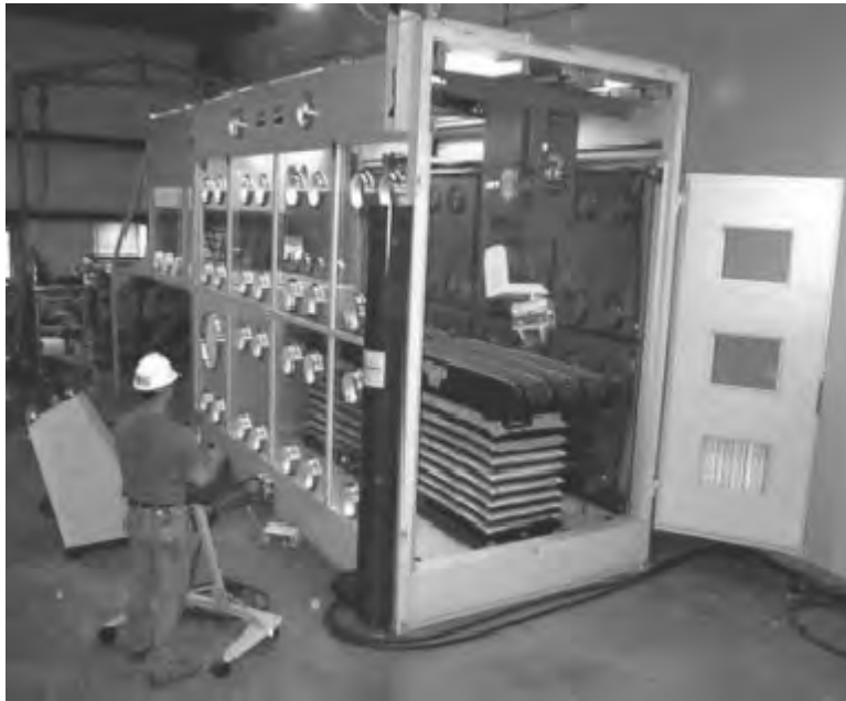
Figure I-20 Example of a Remotely Operated Dismantling System and Inspection Station
