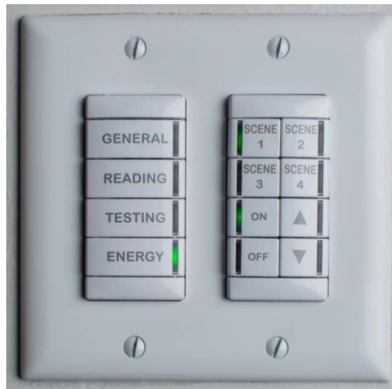
Figure 4. Control station installed in each of the classrooms, with two nLight® nPODM controllers. The controller shown on the left provides SPD control and the controller shown on the right provides light output control. (Image credit: ABL.)
