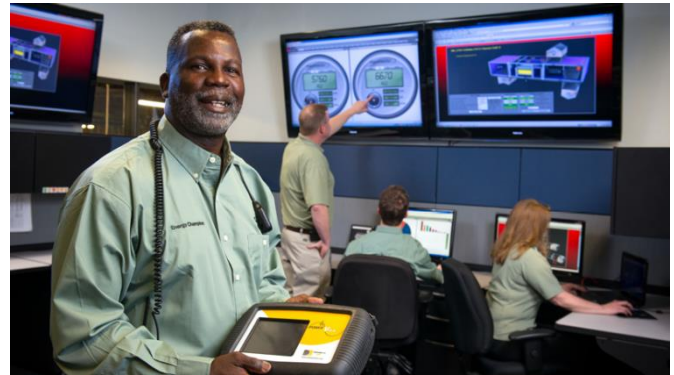
Energy use throughout the Rocky Mount Engine Plant can be monitored and measured from the building management system control room.
