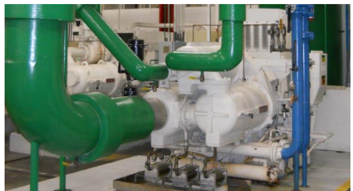
One of RMEP's six centrifugal air compressors, which together meet the compressed air demand in the plant. The six air compressors were identified as one of the plant's significant energy uses (SEUs).
