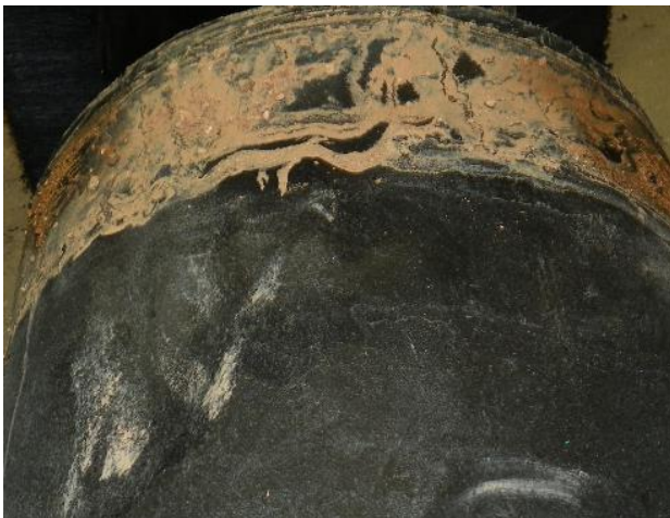
Figure 3: Dirt and mud in an area of the pipe and coupling where fusion between the HDPE should have occurred.
