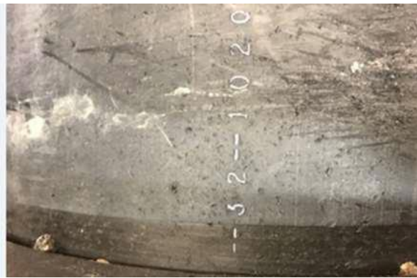
Figure 7: Scraping and the evidence of the print line which is only printed on the outer surface of the HDPE.
