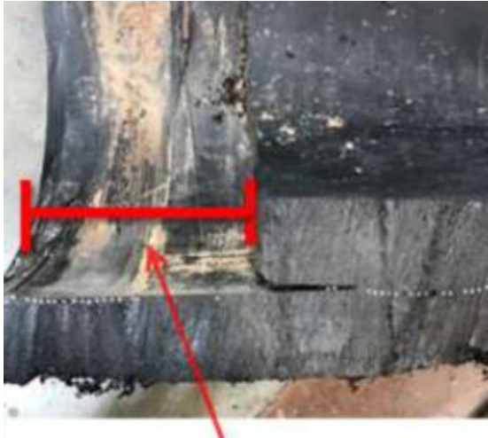
Figure 6: Pipe section is severely miss-stabbed.
