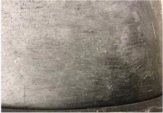
Figure 2: Coupling #1 Pipe surface was scraped.
