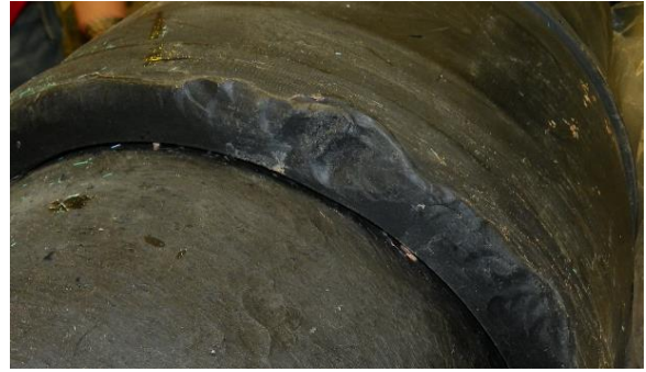
Figure 4: Hammer blows to the coupling indicate that pipe ends were not aligned and force was needed to install.
