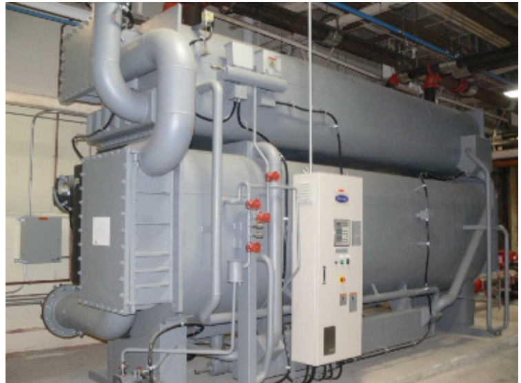
A 400-ton single-stage absorption chiller integrated with three 600 kW reciprocating engines provides hot water for process and space heating. The system is located at a metal fabrication facility in Fitchburg, Massachusetts. Photo courtesy of Northeast CHP Technical Assistance Partnership (CHP TAP).
