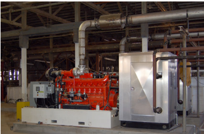
Ammonia/water absorption chiller integrated with a CHP system consisting of two reciprocating engines.
