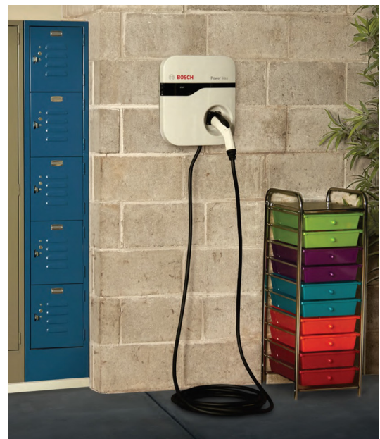
EVSE installation. Source: Bosch
