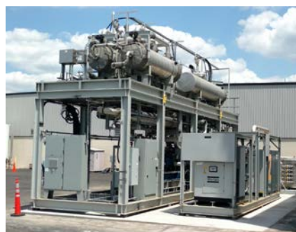
Figure 2: MTR 1MWe Polymeric Membrane System, installed and operational at a coal fired boiler
