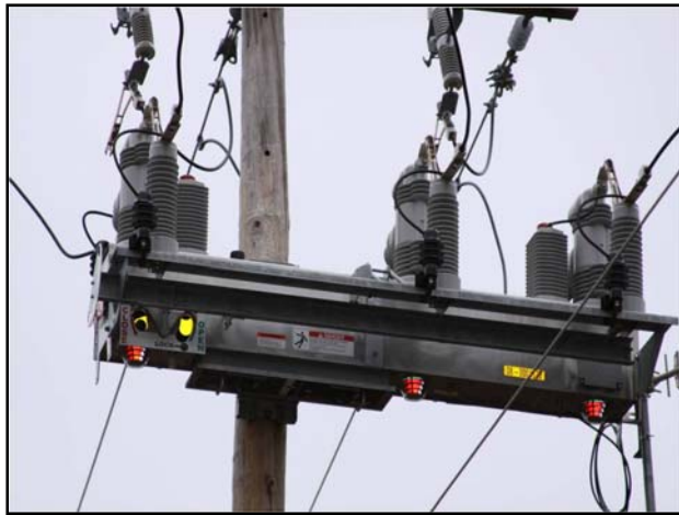
Smart switches installed in EPB service territory
