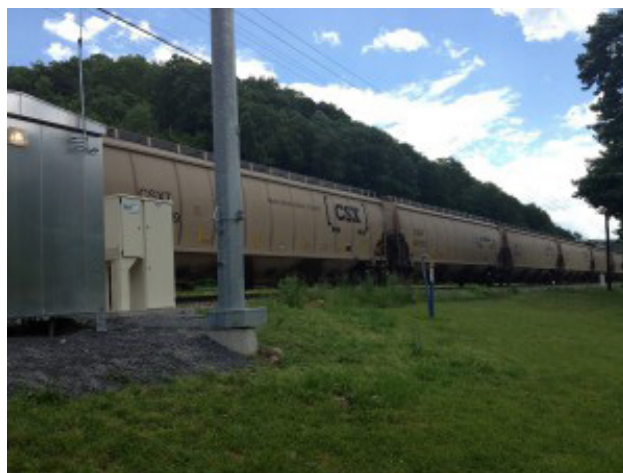
Plug Power fuel cell at railway site
