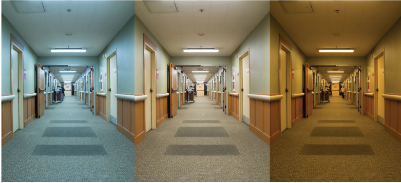
The corridor's new tunable lighting, shown at the morning setting (specified as 6500K at 66% output, left), the afternoon setting (specified as 4000K at 66% output, center), and the nighttime setting (specified as 2700K at 20% output, right).
