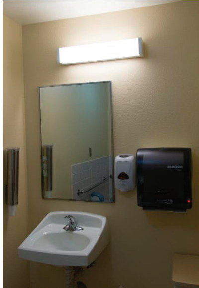
Right: A mirror with integrated LED lighting was installed above the bathroom sink, and a surface-mounted LED luminaire with decorative lens was installed above the toilet area. The amber LED night lighting that was integrated into the railings is also shown.
