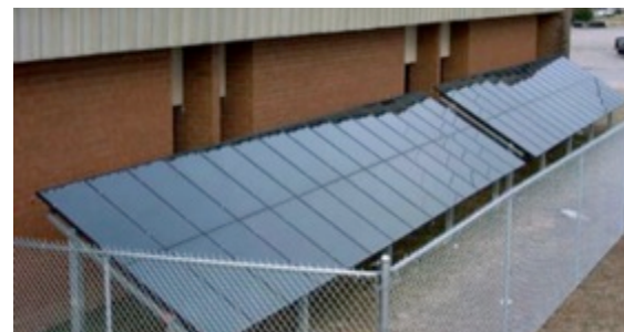
NC Solar Center, NREL 09373
