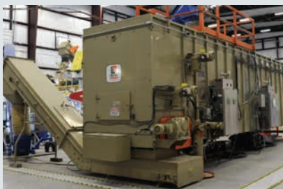
Figure 2. The Biomass Feedstock National User Facility (BFNUF) is the most complete feedstock preprocessing R&D facility in the world. Located at Idaho National Laboratory, BFNUF was developed to help overcome key technical barriers facing the U.S. bioenergy industry by investigating advanced feedstock supply and logistics, analysis and sustainability, preprocessing, and characterization. Photo courtesy of Idaho National Laboratory.
