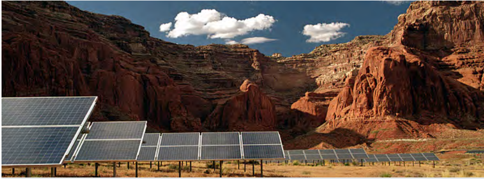
This PV array in Lake Powell, Utah provides electricity to Dangling Rope Marina, replacing diesel-fueled power generators. Photo Courtesy: Department of Energy
