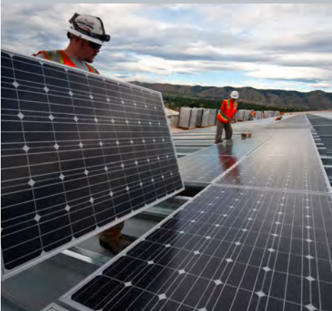
Crews install PV panels at the National Renewable Energy Laboratory's Research Support Facility. Photo Courtesy: Department of Energy
