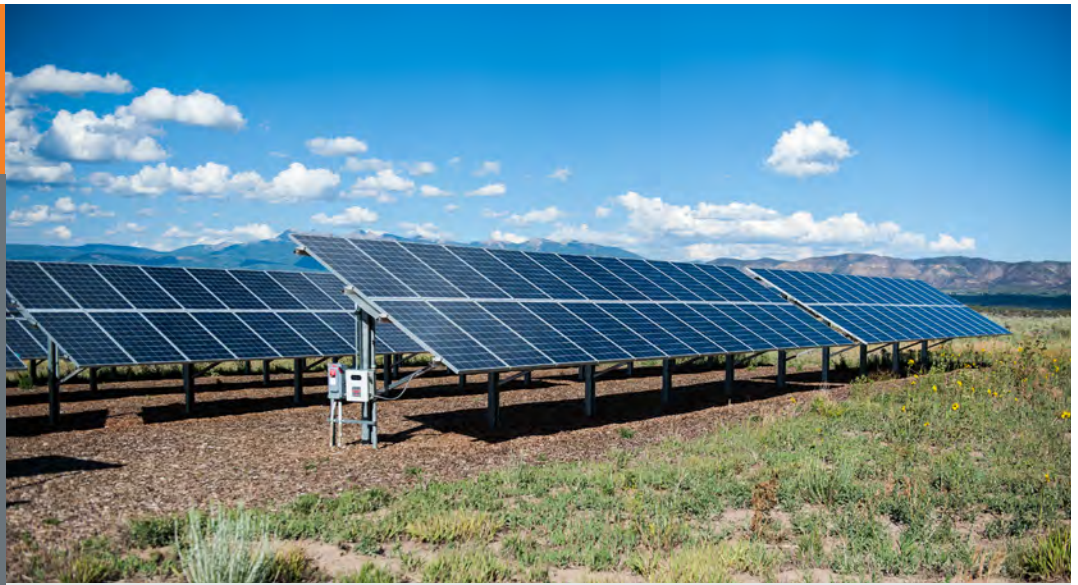
Mesa Verde National Park in Colorado is the home of this PV array, where it provides energy for the visitor center. Photo Courtesy: Department of Energy
