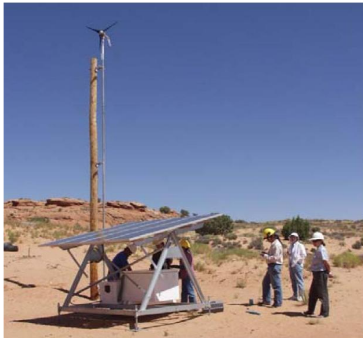
Figure 1. 880-Watt Hybrid System in Monument Valley, Utah
