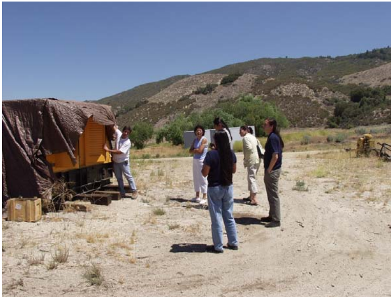
Figure 7: Propane generator will be used as a back-up energy source for the micro-grid hybrid system.
