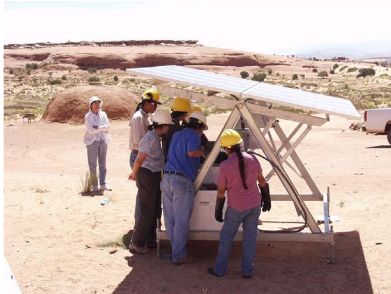
Figure 6: NTUA electricians and Sandia interns performing O&M.
