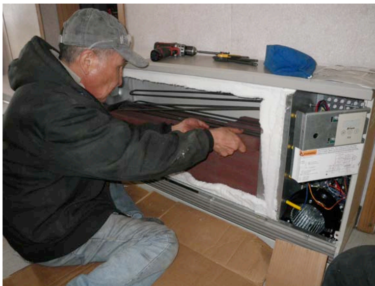
Technician Wassilie Lupie installs an ETS device in a home in Tuntutuliak, AK.
