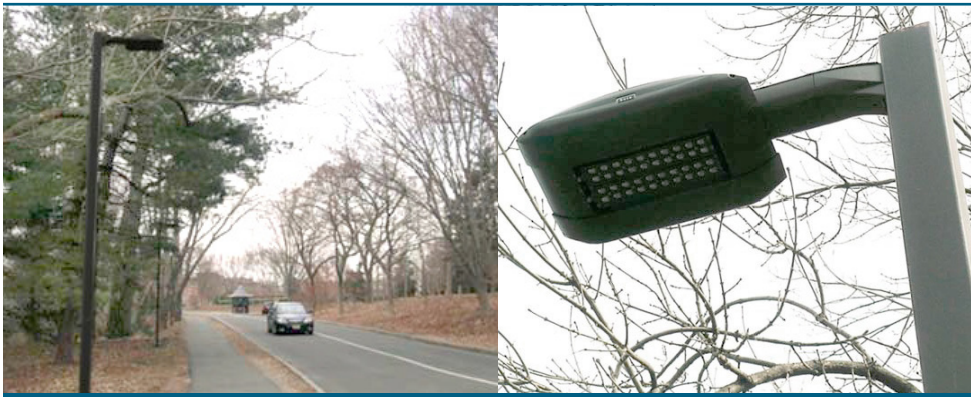
New LED luminaires along Elm Drive (left), and a close-up view (right). Photo: Pacific Northwest National Laboratory.
