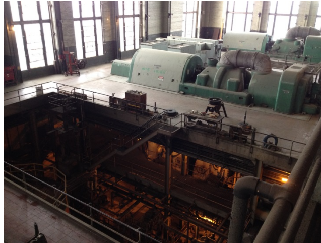
Figure 1.2. Idled Mistersky generators, December 2013. Photo: PNNL
