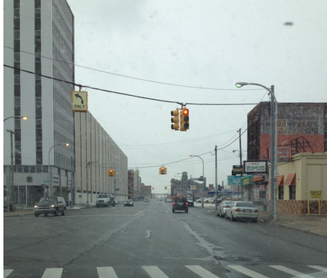
Figure 1.3. Street lighting circuit operating during daytime hours due to an absence of staff to turn it off. Photo: PNNL
