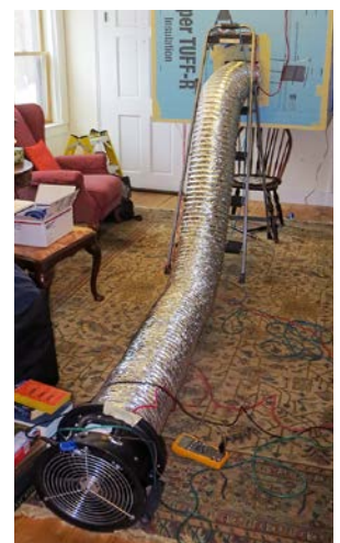
Figure 1. Flow testing configuration measured flow rates that were 50%–80% of manufacturer-listed rates.
