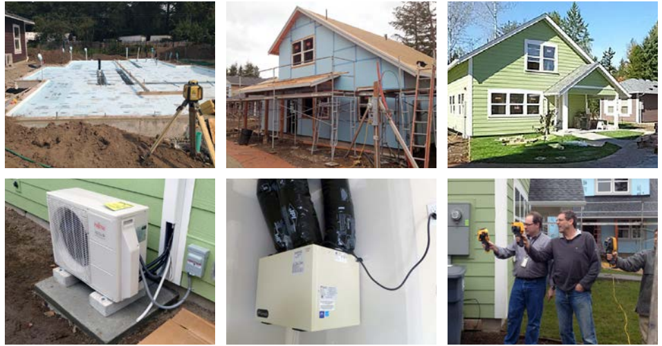
From left, top: R-15 slab; foam sheathing; “The Cottage,” a 3-bedroom, 1,267-ft 2 home. From left, bottom: DHP outside unit, HRV unit in mechanical room, infrared-guided blower door testing and training by BA-PIRC partners.
