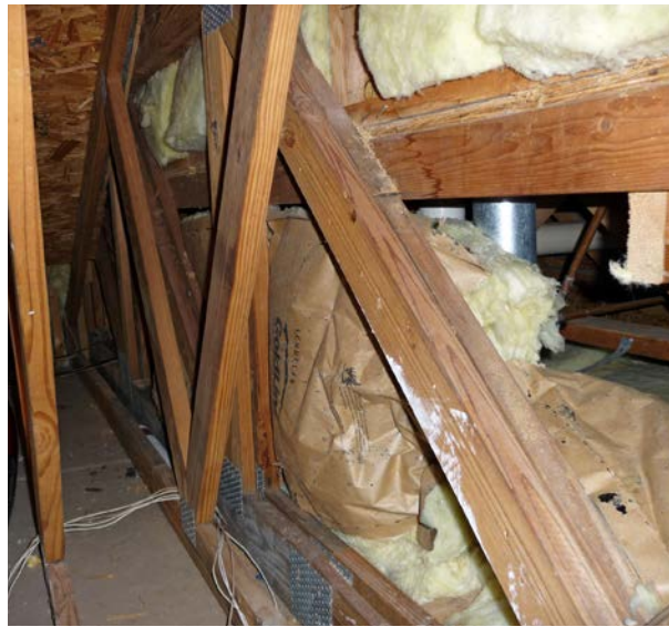
Figure 2. Visual inspection is important to determine the existence of wind washing, the resulting problems, repair strategies, and the potential benefit of the repair. The image on the left shows poorly installed batts and a pathway in a floor cavity open to the attic. Field tests can also be useful. These tests include infrared (IR) scans of house surfaces (see sidebar), house and duct leakage tests, and pressure mapping.
