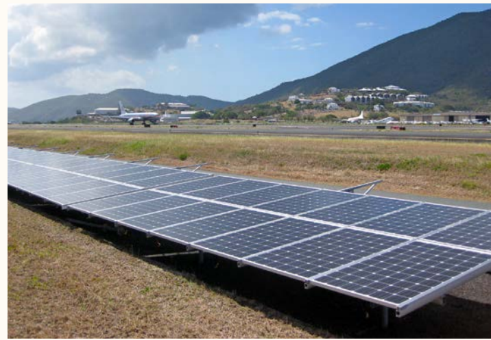
A 448-kW PV system installed at the Cyril E. King Airport on St. Thomas in April 2011. Photo by Adam Warren, NREL 18953
