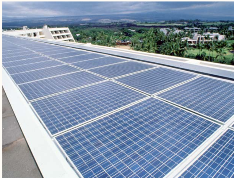
The rooftop solar PV on Hawai‘i’s Mauna Lani Bay Hotel generates 75 kW of electricity. Photo from SunPower, NREL 06430
