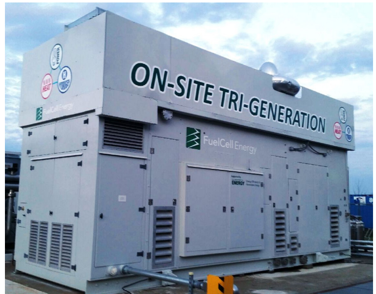
The combined heat, hydrogen, and power system, which includes a 300 kilowatt fuel cell and a hydrogen booster, being installed at a manufacturing facility in Torrington, Connecticut.
