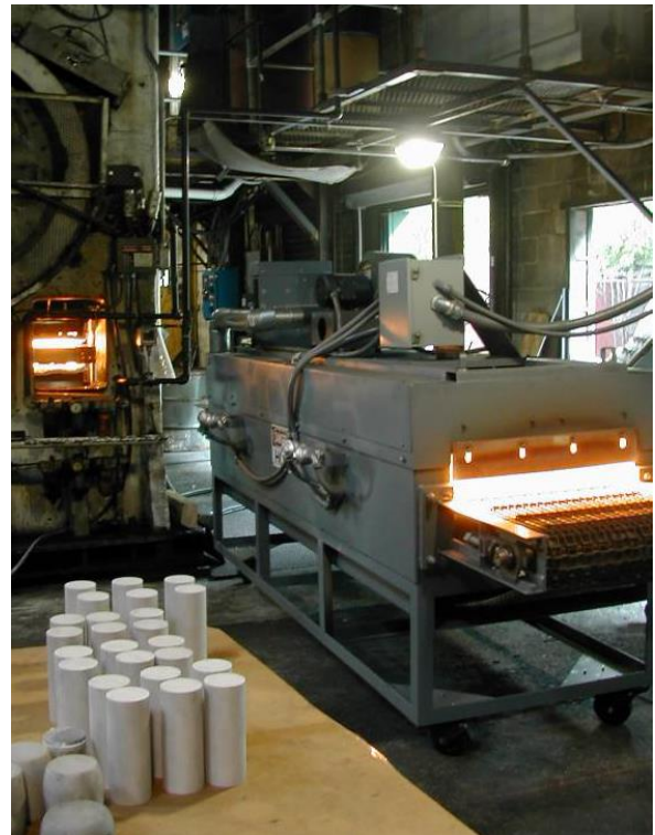
Figure 4 - Continuous-belt IR heating furnace installed at Queen City Forging Company, Cincinnati, Ohio [10].
